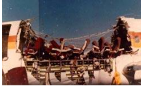
Figure 9. An example of corrosion fatigue due to the stresses created by buildup of crevice corrosion products inside the lap joints followed by cyclic loading (KSC, 2014 and Roberge, 1999).
