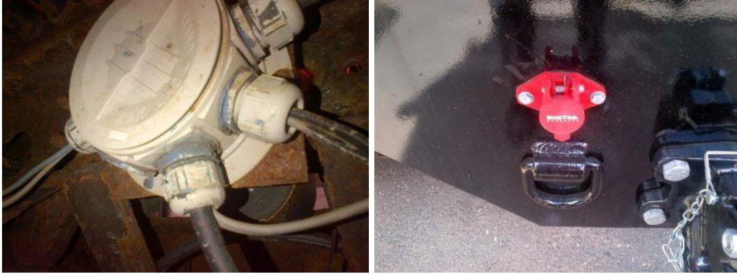
Figure 105. Electrical components in bad condition (left); ConnDOT requires body builders to provide sealed connections and plugs and use dielectric grease on them (right) (Chupas, 2014).
