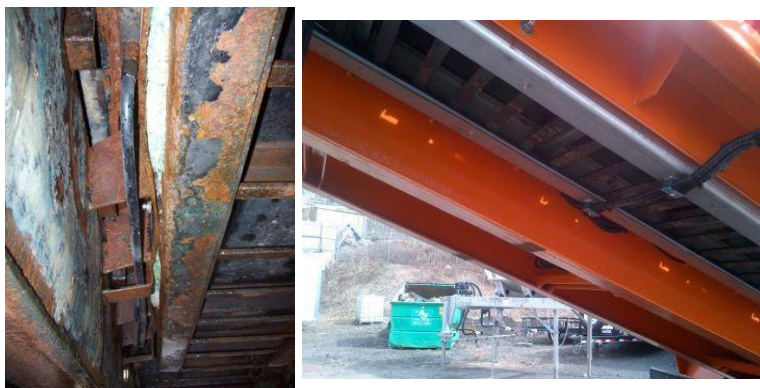
Figure 100. A 2007 corroded body (left), and a 2012 protected body by using a mix of weathering steel (Cor-Ten) and stainless steel (right) (Chupas, 2014).
