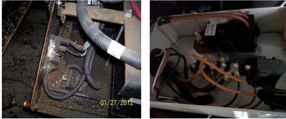
Figure 45. A relay and circuit breaker for spreader controls; mounted in the battery box (left), enclosed box inside the cab of the truck (right) (Smith, 2014).
