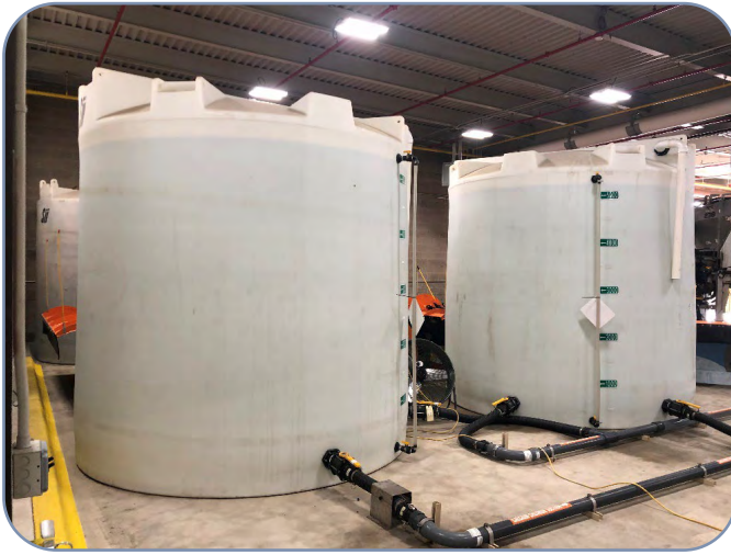
Effectively constructing and managing liquid chloride storage tanks is essential for transportation agencies that deice roads in wintry weather.
