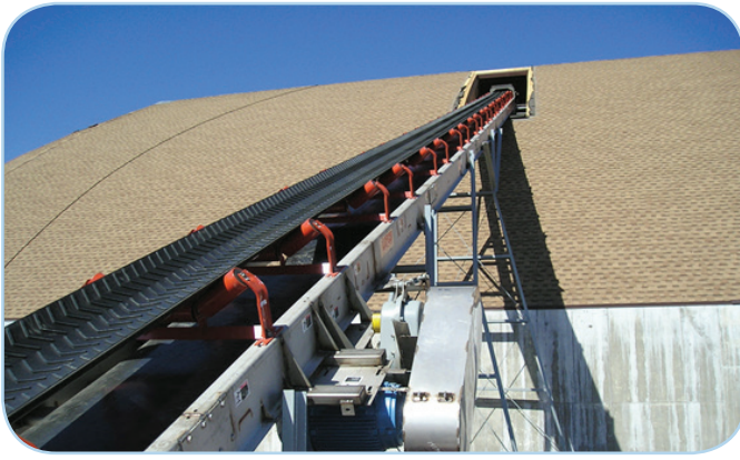
Conveyor systems that fill a salt storage facility from its highest point maximize the capacity of the facility and are safer than simply pushing salt into a stockpile.
