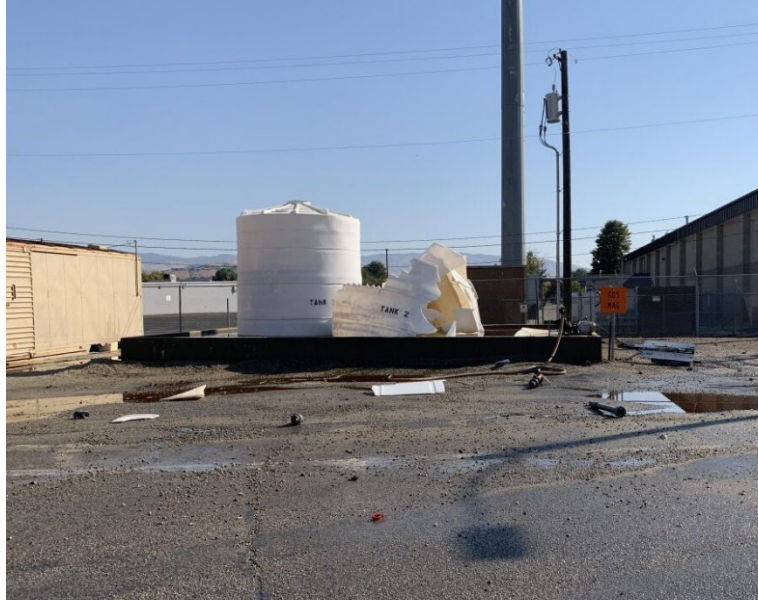
Figure 23: Storage Tank Rupture
