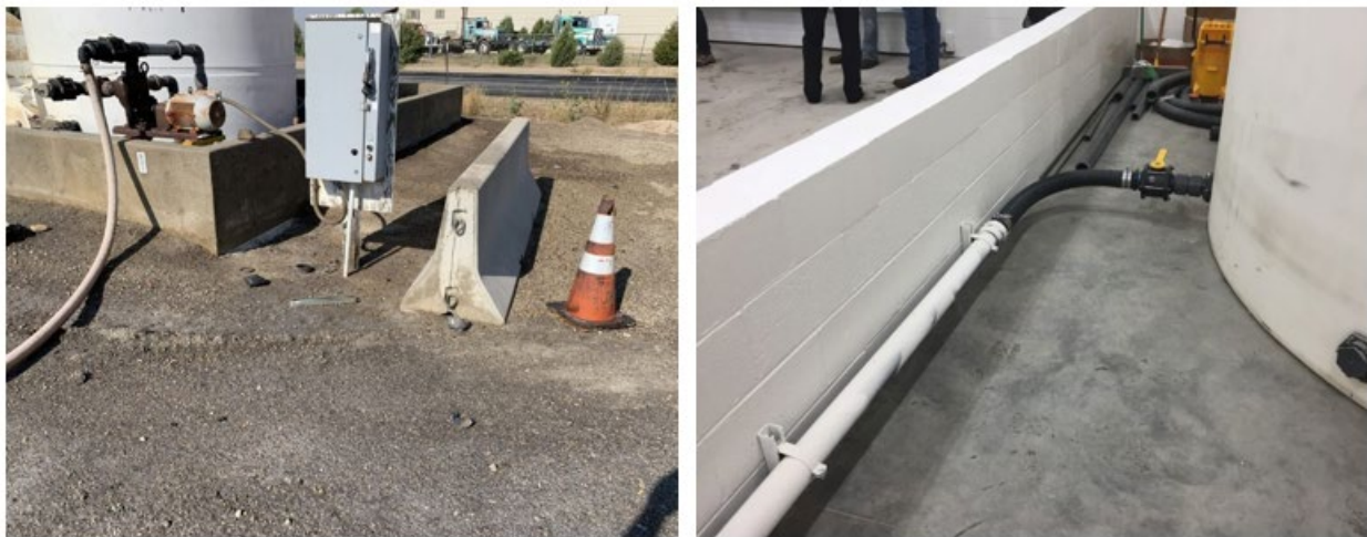
Figure 21: Liquid Deicer Storage and Pump System Secondary Containment Concrete Wall
