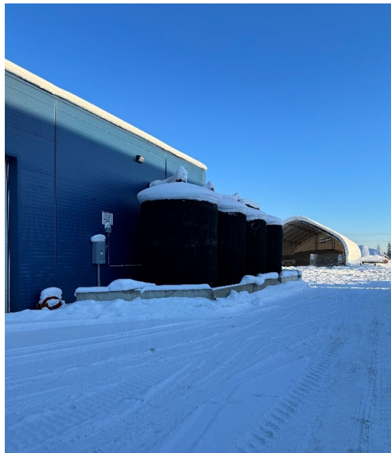
Figure 13. Liquid Deicer Storage Tanks
