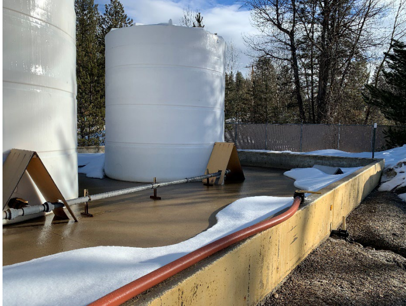
Figure 22. Coverings for System Plumbing
