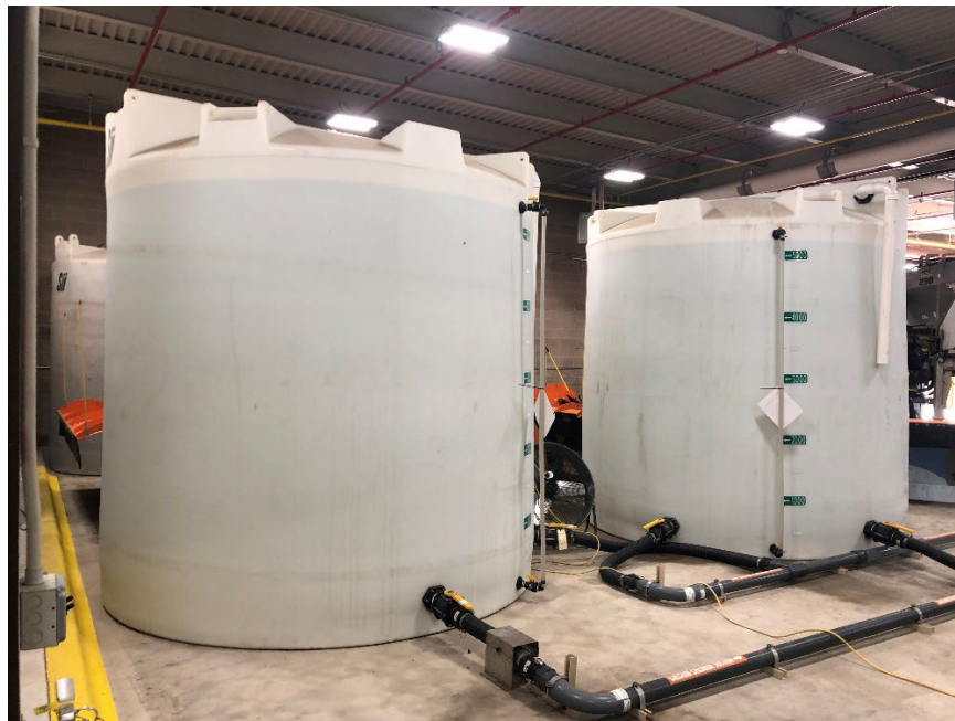
Figure 19. Liquids Storage Tanks
