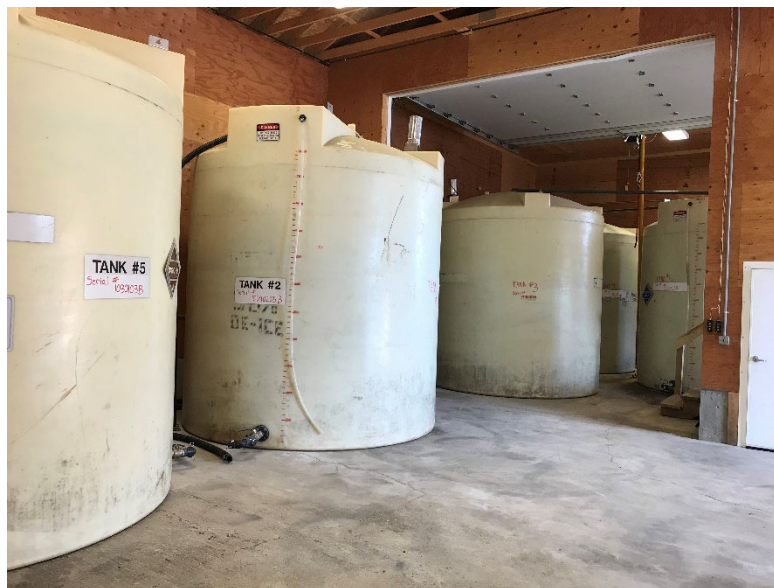
Figure 28: Liquid Deicer Storage Tanks
