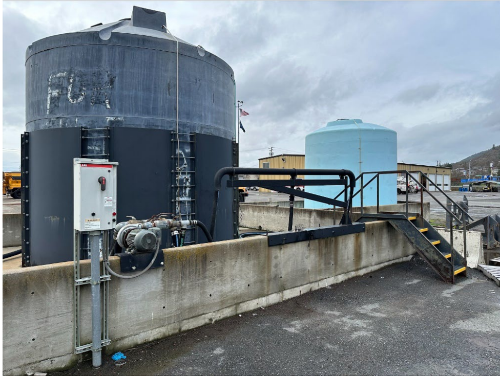
Figure 33. Storage Tank with Secondary Containment Retention Wall
