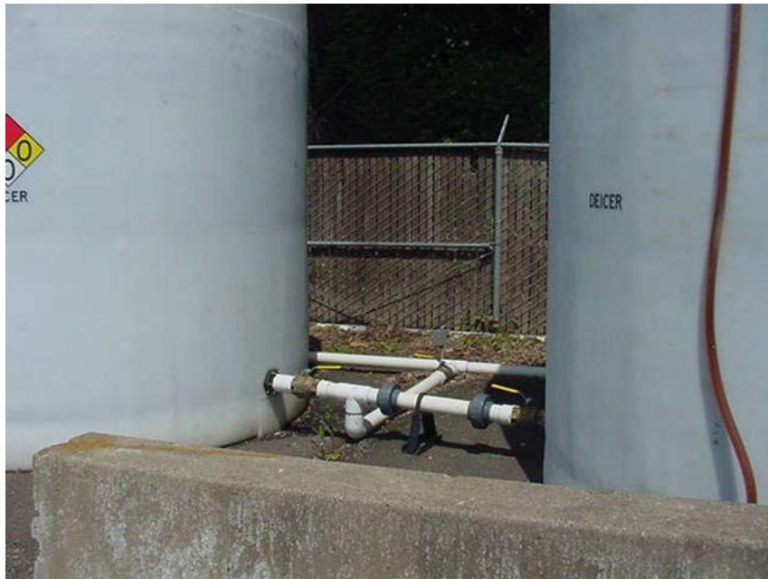
Figure 32: PVC Plumbing of Liquid Deicer Storage Tanks.
