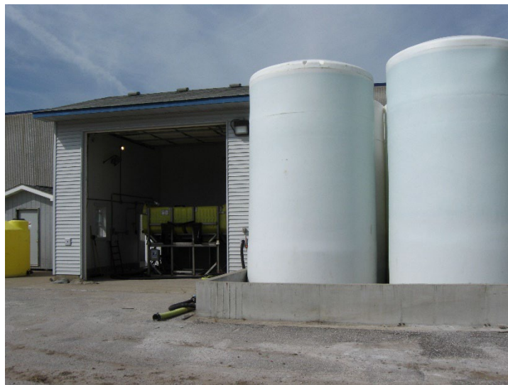
Figure 20. Iowa DOT Liquid Deicer Storage Tanks
