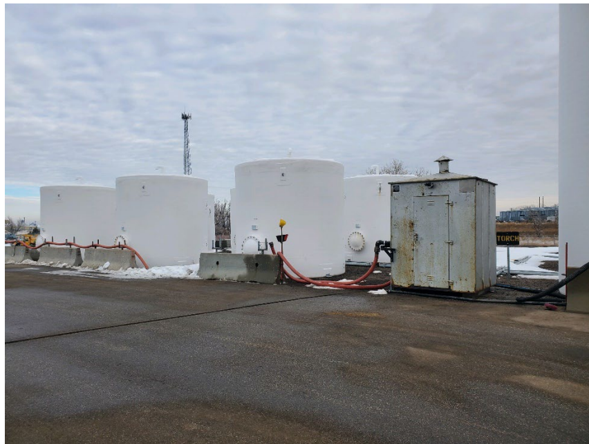
Figure 30. NDOT Tank Farm and Pump House
