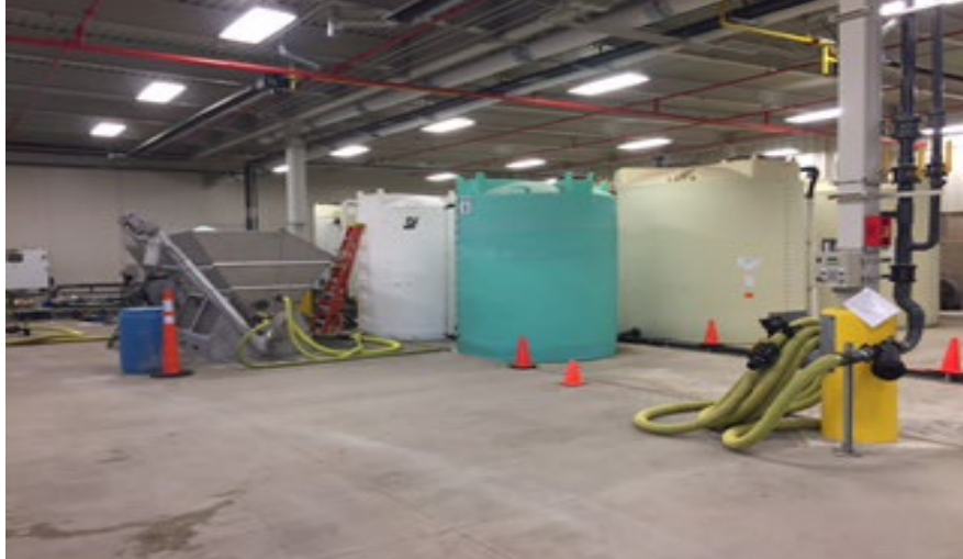
Figure 18. Liquids Manufacturing Room - Storage Tanks
