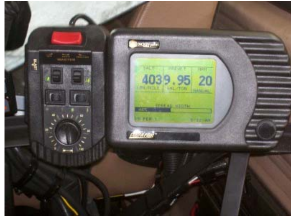
Figure 4-1 Controller in a spreader truck cab with speed simulator display.
