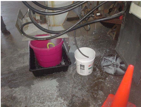
Figure 4-10 Large plastic tub inside a mason tub for catching small amounts of discharged solid material.
